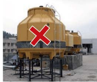
No need cooling water tower
